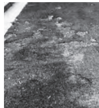
A road showing signs of salt and water impacts. Source: DIPNR
