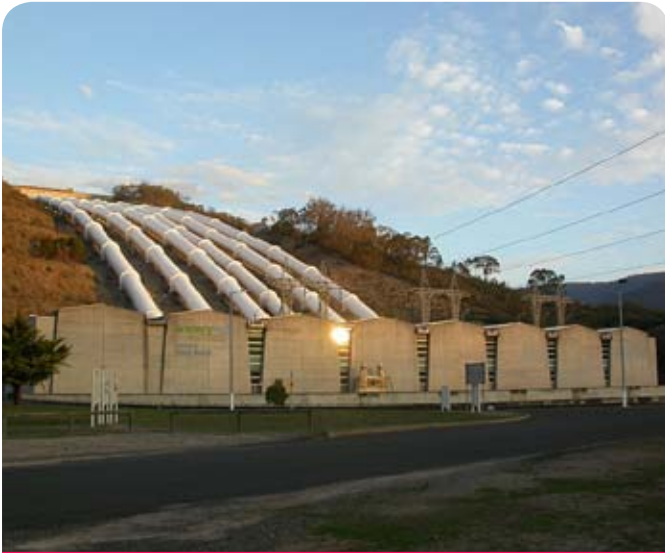
Tumut 3 Generating Station is one of three hydroelectric power stations on the Tumut River in NSW. It is part of the Snowy Mountains Hydroelectricity scheme. Source: Image by Colin Henein/GFDL Wikimedia Commons
