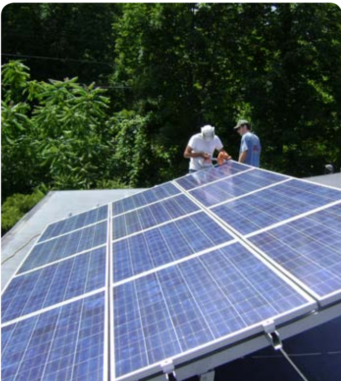
Two workers installing a tilt-up photovoltaic array on a roof. Source: Labraun90/Wikimedia
