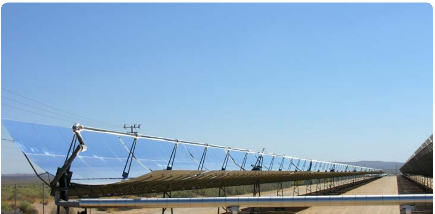
This is a parabolic trough solar thermal electric power plant located at Kramer Junction in California. Source: kjkolb/Wikimedia Commons
