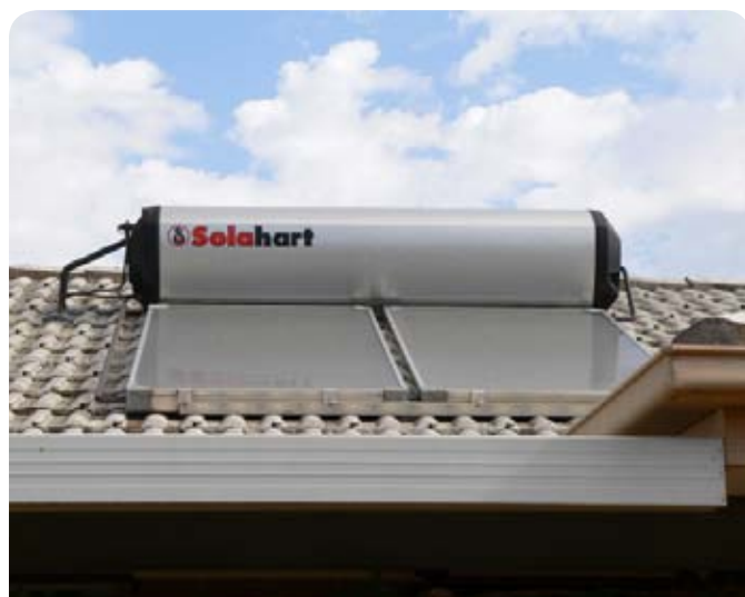
A Solarhart brand solar hot water panel and integrated tank on a house roof in Australia. Source: Fairv8, Wikimedia Commons
